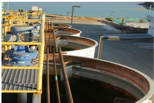
Water tanks which are part of the water treatment process at the mine
